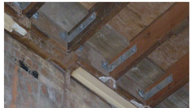
Figure 5. Wall to floor strengthening bolted solutions using steel rods bolted to steel angles
