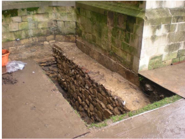
26 Figure 6. Part of the exposed foundation at the west corner of the southwest transept.
