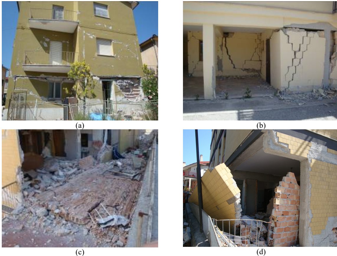
Figure 4: Masonry infill damage, (a) separation between infill and frame, (b) in-plane damage, (c) out-of-plane collapse, (d) out-of-plane failure.
