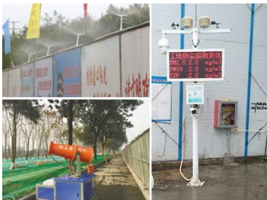
Figure 21 - Dust removal and monitoring system
