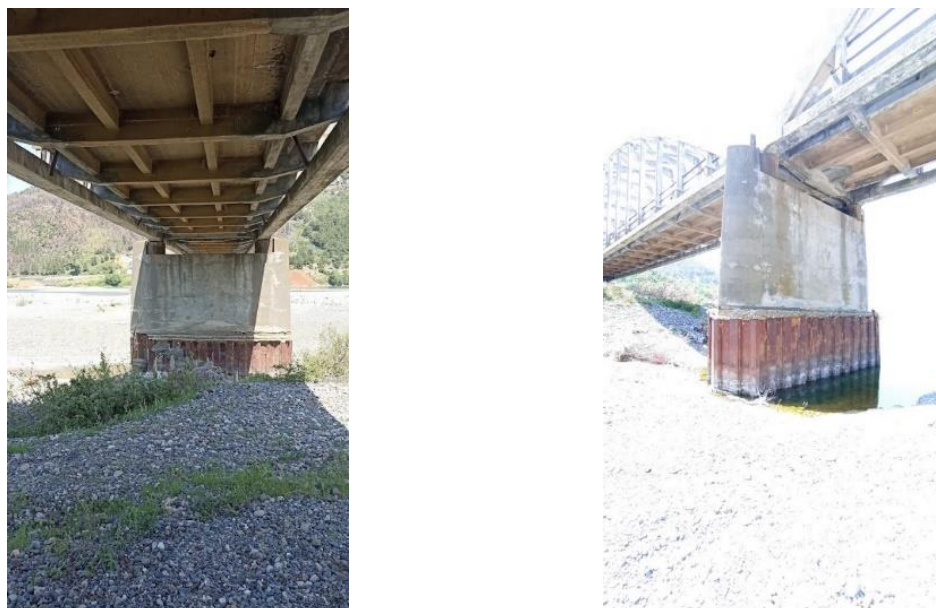
Figure 51 – Scour problems in the foundation of the Ura e Zogut bridge
