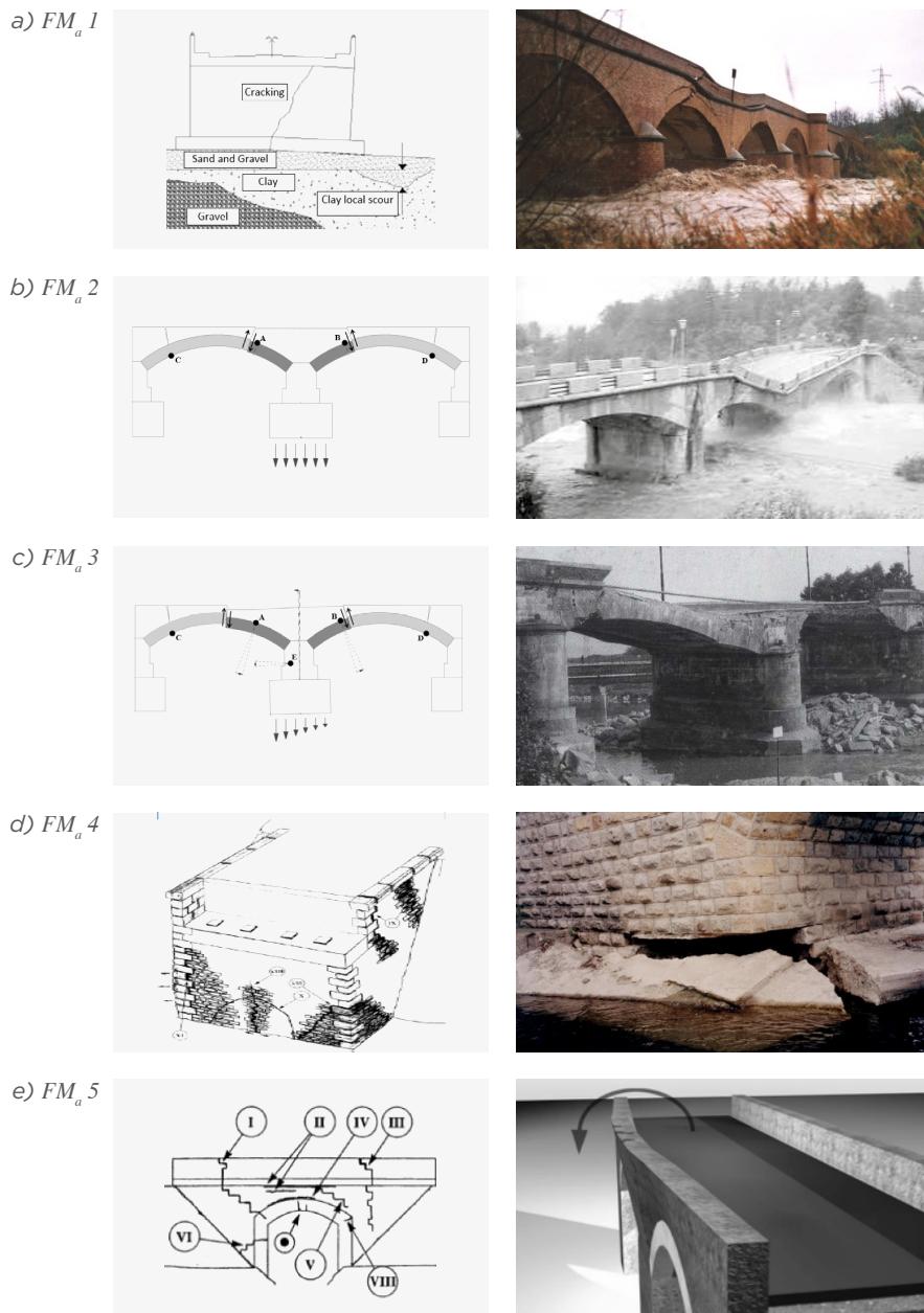
Figure 10.10 Failure modes of masonry arc bridges a) Fragmentation of a pier, (FHWA, 2011); b) Symmetrical, in-plane failure mode, (Zampieri, et al., 2017); c) Non-Symmetrical, in-plane failure mode (Zampieri, et al., 2017); d) Failure mode related to fragmentation of an abutment, (SÉTRA, 1996) e) Out-of-the -plane failure and spandrel wall displacement, (SÉTRA, 1996);
