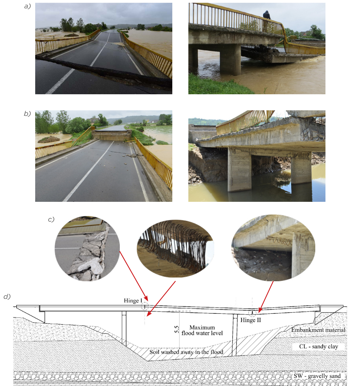
Figure 10.16 Bridge failure forensics
