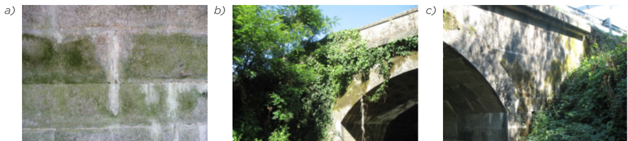
Figure 9.25 Damages - environmental and chemical actions, (Infraestruturas de Portugal, 2007) a) Water flowing, efflorescence, stalactites and vegetation, on the arch intrados; b) Vegetation and black films (the southwest face on the spandrel wall); c) Moss and lichens (the northwest face on the spandrel wall)
