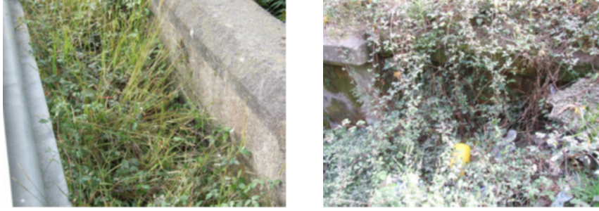
Figure 9.26 Obstruction of the drainage system at the deck level, (Infraestruturas de Portugal, 2007)
