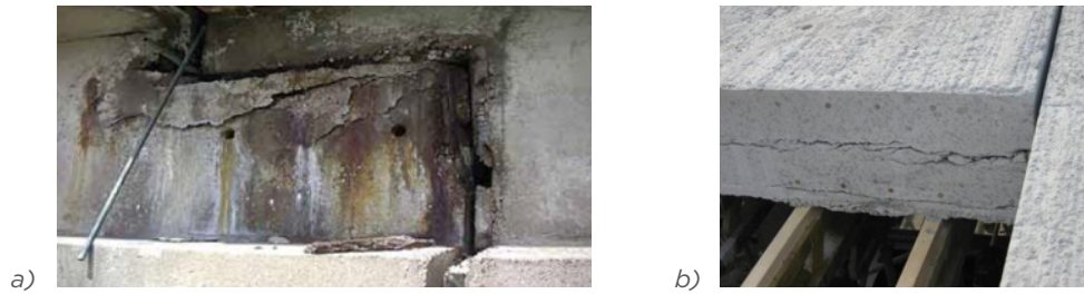
Figure 7.4 Examples of observations that affect vulnerable zones a) Chloride induced corrosion in a half-joint, ( CIRIA, 2017 ); b) Delamination due to ASR in a deck slab (affecting the shear resistance), ( Larsen, 2009 )
