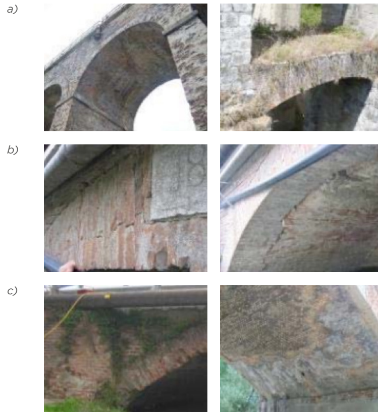
Figure 7.6 Typical defects of masonry arch bridges, from (Zampieri, 2014)
