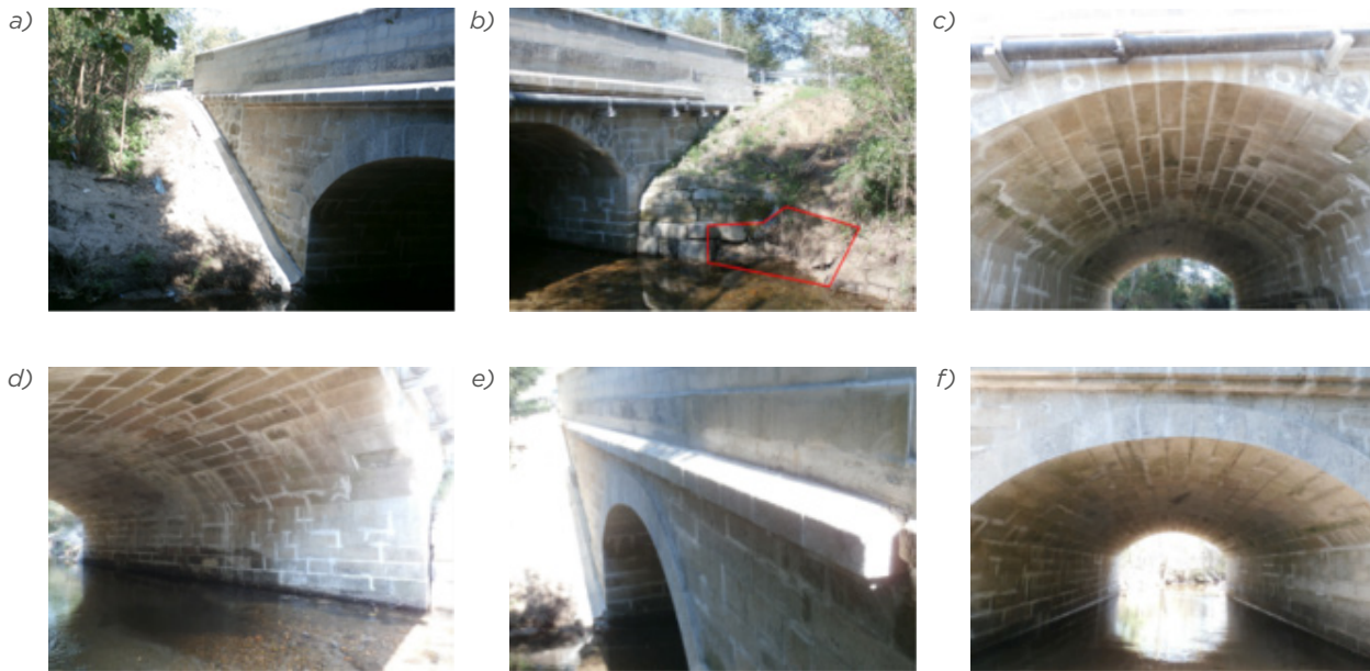
Figure 9.32 The bridge elements/sections after the rehabilitation (Infraestruturas de Portugal, 2015): a) spandrel walls (the north-western part of the bridge); b) spandrel walls (the north-eastern part of the bridge) and lack of material in the embankment; c) intrados of the arch view from east; d) north-eastern part of the arch intrados and abutment; e) southwest view of the bridge; f) west view of the arch intrados.
