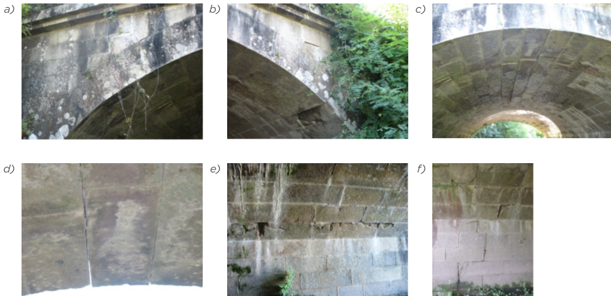
Figure 9.27 Damages associated with mechanical actions, (Infraestruturas de Portugal, 2007):
