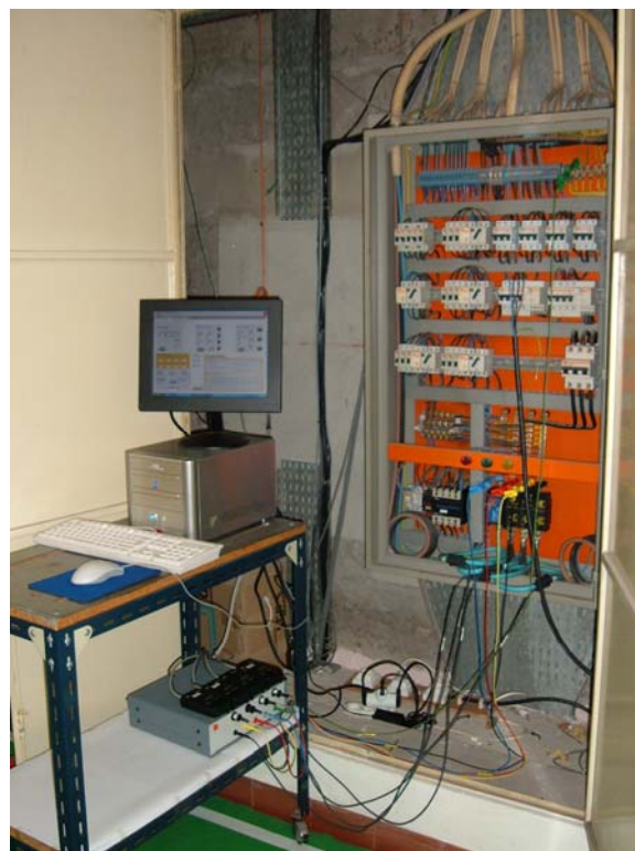
Figure 1 - Developed Power Quality Monitor in an electrical panel
