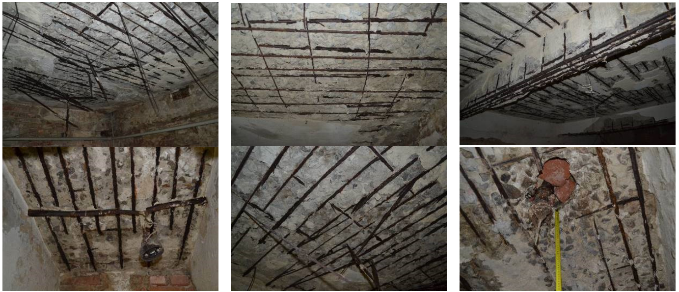
Figure 5. General view of the sub-basement slab: corrosion damage to the reinforcement bars of the floor slabs and destruction of the concrete protective layer.
