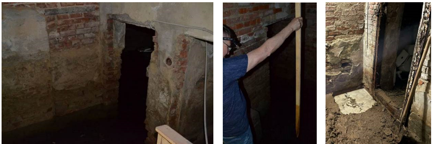
Figure 4. Flooding of the school basement rooms: destruction of the lime matrix in the joints and moisture saturation of the brick structures in the basement.
