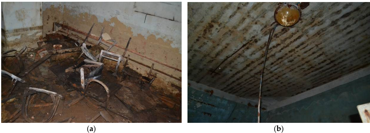
Figure 1. Primary defects of the inspected basement shelter that has been out of operation: (a) damage to the finishing layer and erosion of the shelter's wall and floor structures due to prolonged water exposure and saturation; (b) corrosion damage to the reinforcement of precast reinforced concrete roof panels, formation of corrosion-induced crack, deterioration of protective plaster, and efflorescence.
