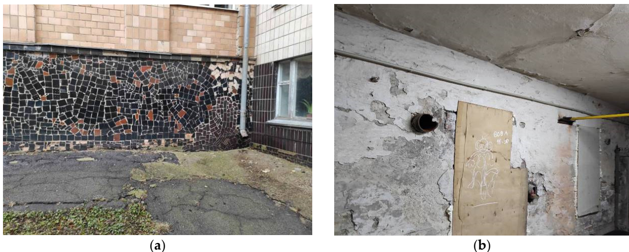
Figure 6. Specific defects of the academic building: (a) damaged pavement around the building, allowing water to flow through the wall and flood the basement; (b) deterioration of the basement wall surfaces due to plaster damage and efflorescence formation.
