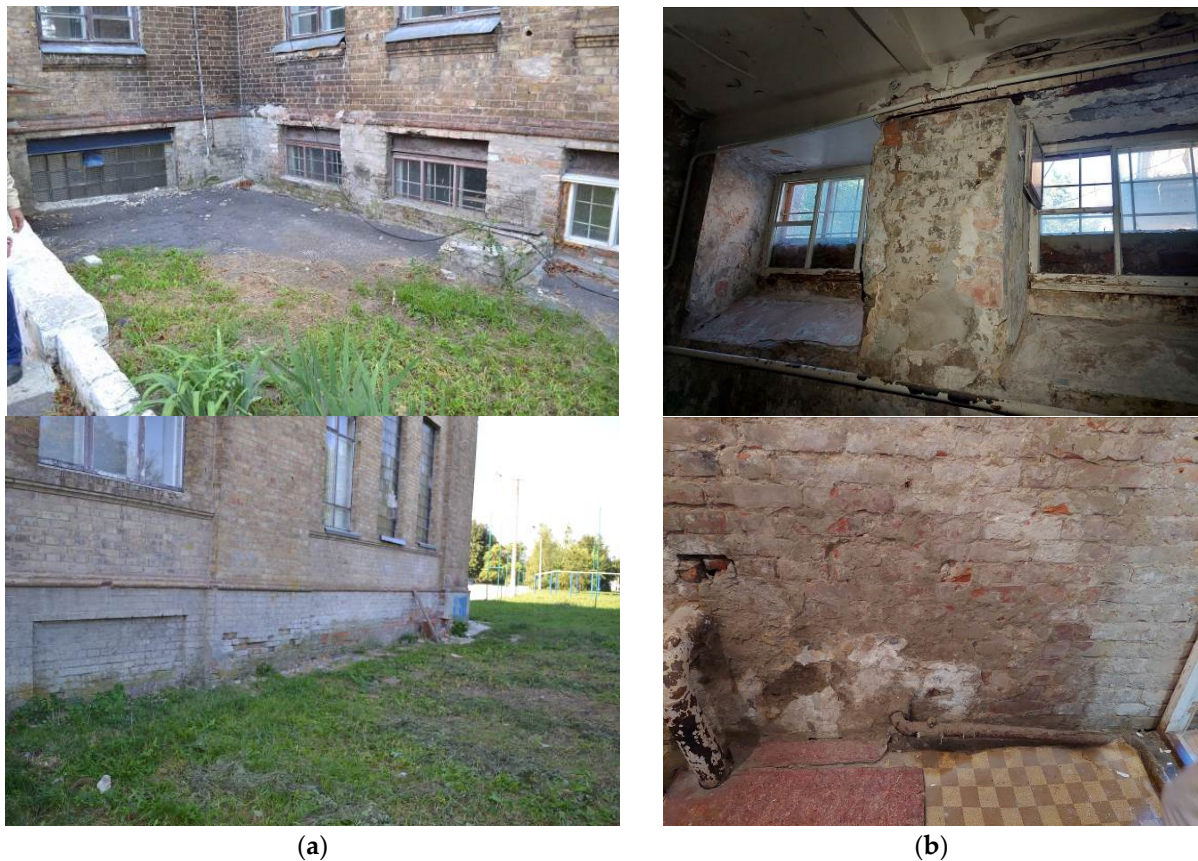
Figure 2. Relevant defects of the inspected historical gymnasium building in the Poltava region: (a) the pavement around the building is in an unfit condition, and the site grading promotes the accumulation of atmospheric water, leading to its localized infiltration into the foundation base; (b) deterioration of the interior wall surfaces in the basement due to capillary moisture rise, resulting in plaster damage and efflorescence formation.
