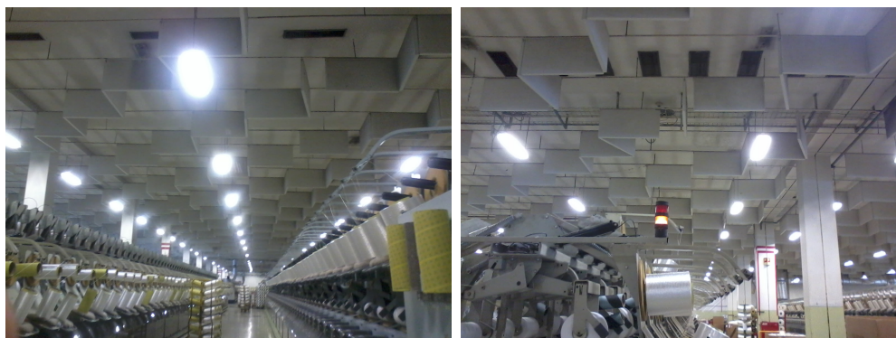
Figure 3.3: Air ventilation grids with dimensions 0.15 m x 0.85 m (left panel) and 0.35 m x 0.85 m (right panel) on the ceiling of Nave 2.
