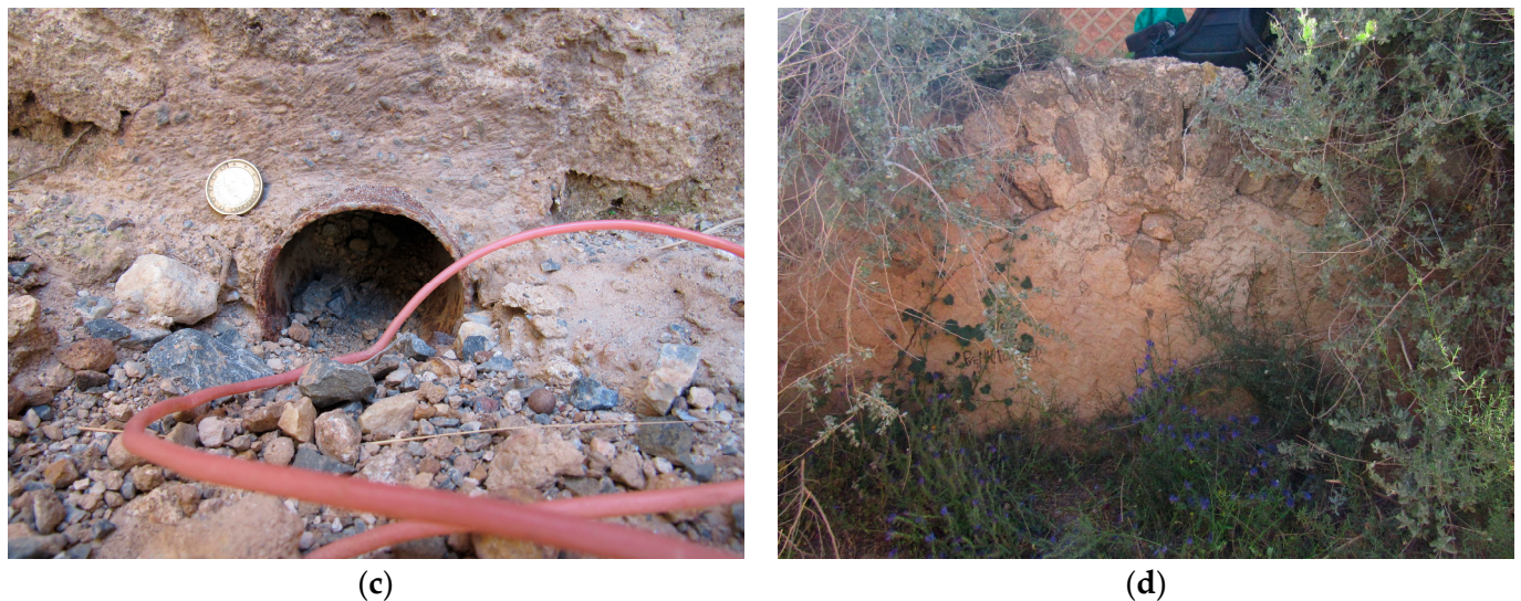
Figure 2. Current conservation state of the Castle of Lanjarón: (a) state of metallic elements in the castle; (b) alveolized limestone ashlar; (c) blocked drainage tube; (d) significant plant growth on structural elements hides a masonry arch.
