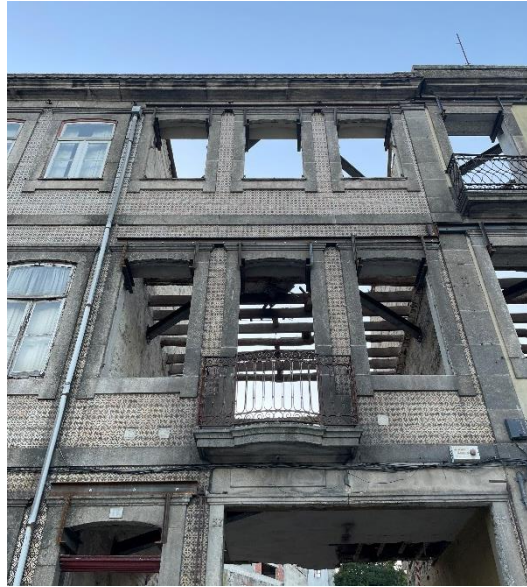
Figure 2.4. Degraded timber floor in an existing building in Porto (PT).
