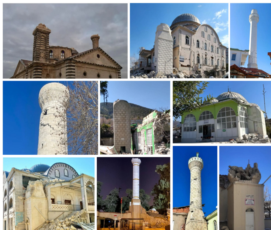
Figure 6. Examples of minarets damaged in the 2023 Türkiye earthquakes [28].
